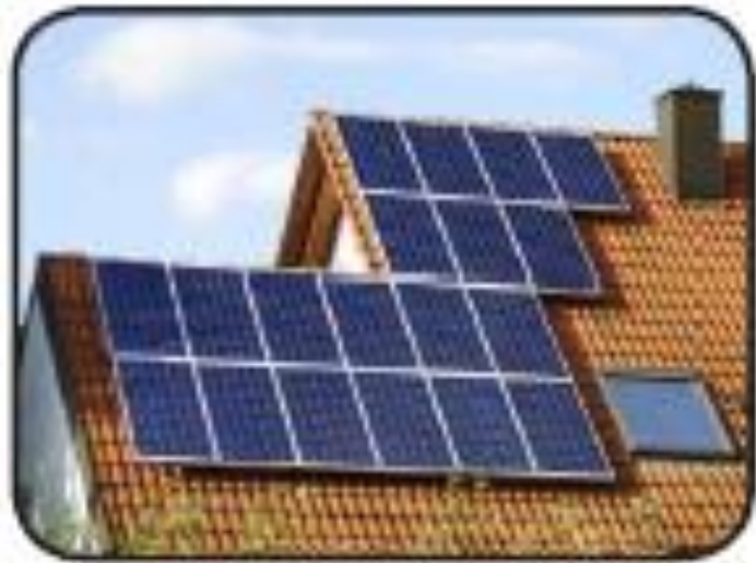
Solar panels collect energy from the Sun.
